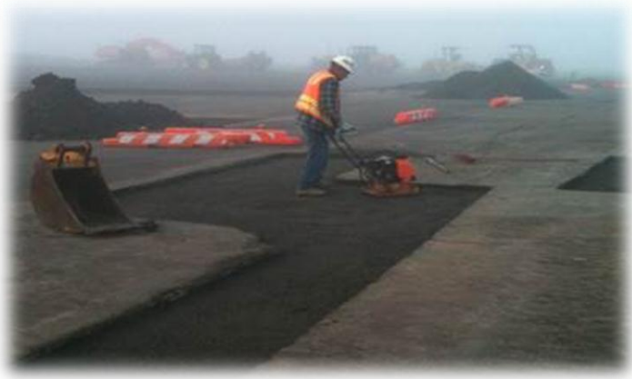
Patch Repair; Rock compaction at Hillsboro Photo credit: James Kirby, Jr., PE
