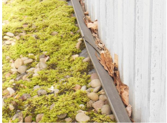
Membrane shrinkage has pulled edge flashings away from structure.
