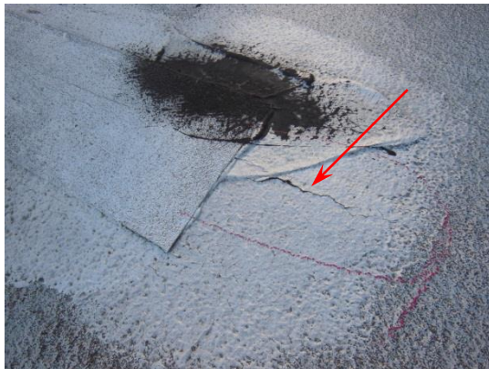
Membrane split has extended beyond previous repair patch.
