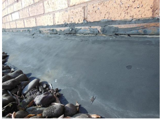
Membrane shrinkage has pulled base flashings away from the wall substrate.
