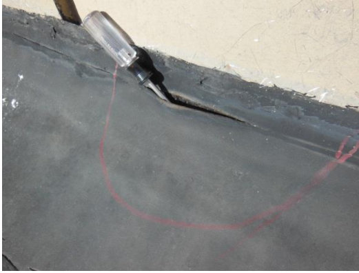
Membrane shrinkage has pulled base flashing from substrate and top edge is open.
