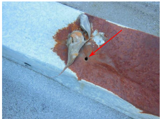
Sheet metal curb cover is significantly rusted and puncture can allow water entry.
