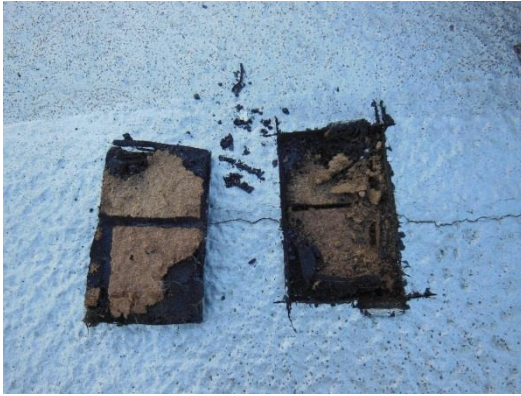
Core sample taken at membrane split reveals splits are occurring at joints in the single layer of wood fiber insulation.
