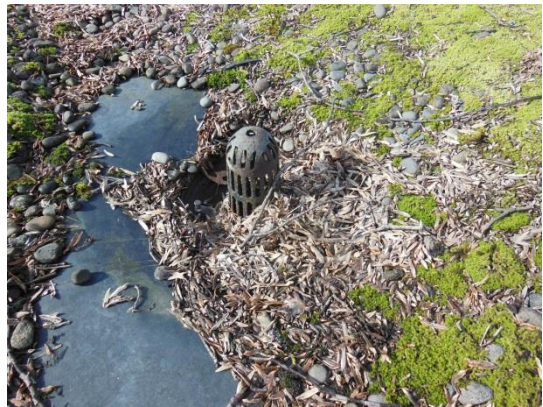
Roof drains are restricted by organic debris (typical condition).
