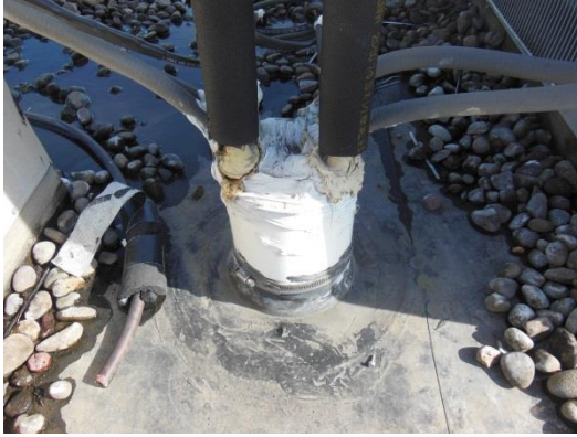
Utility line penetration is poorly detailed and is sealant dependent.
