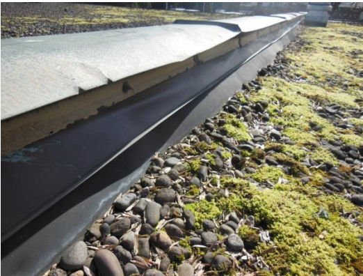
Membrane shrinkage is pulling base flashings away from expansion joint curb.
