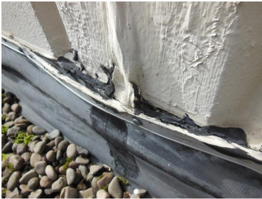
Base flashings are poorly detailed at vertical joints in concrete wall.
