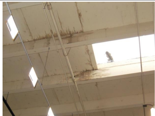
Ongoing leaks have resulted in localized deck deterioration.
