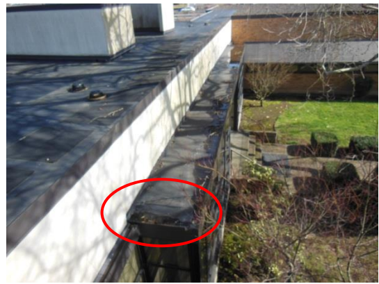
Overview of Roof Area Q. SW corner has been a chronic leak location.
