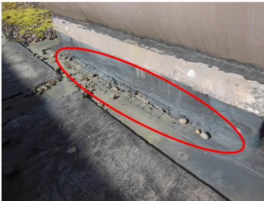
Curb flashing has failed, allowing active leakage at HVAC unit.
