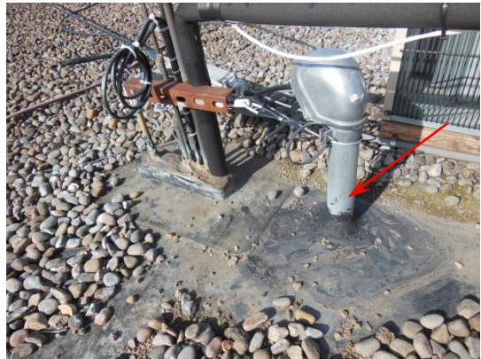
Conduit penetration lacks a proper flashing.
