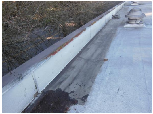
The roof membrane at each of the four drain locations has been repaired/overlaid with an APP modified bitumen membrane.
