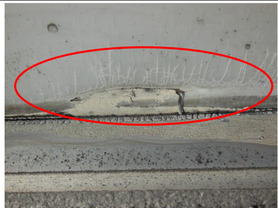
Improper application of elastomeric sealant at edges of acrylic domes has resulted in spider web cracking in the domes.
