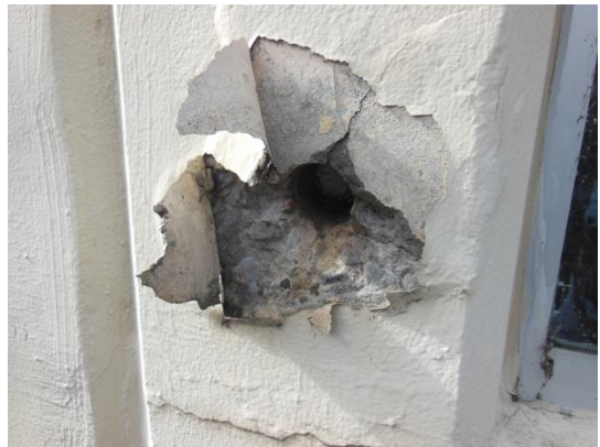
Abandoned through-wall penetrations are poorly sealed.
