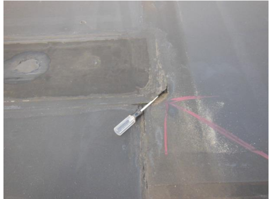
Void in membrane patch can allow water entry.
