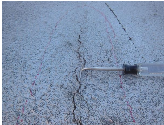
View of additional membrane splitting in the field of the roof.
