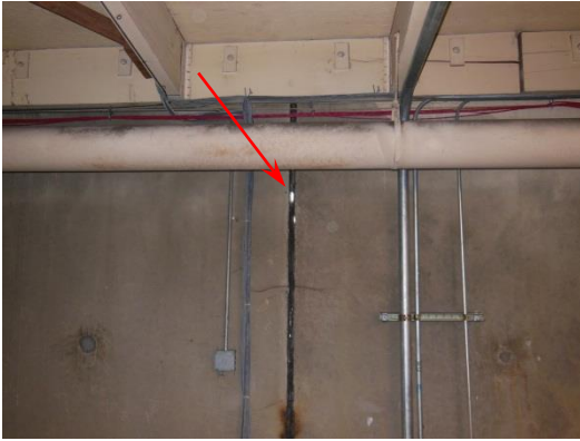
Interior view of vertical expansion joint reveals sealant failure, as daylight is visible from the inside.
