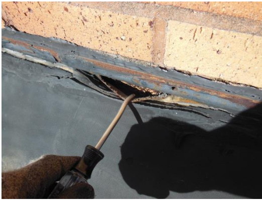
Top edge of base flashing is open.
