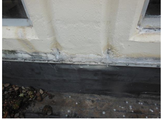
Base flashing termination is less than optimum and is sealant dependent.
