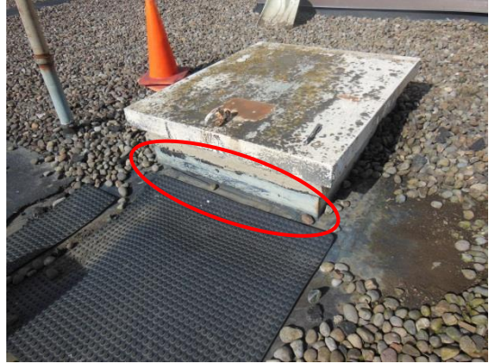
Roof hatch lacks a vertical flashing and horizontal strip flashing has failed.
