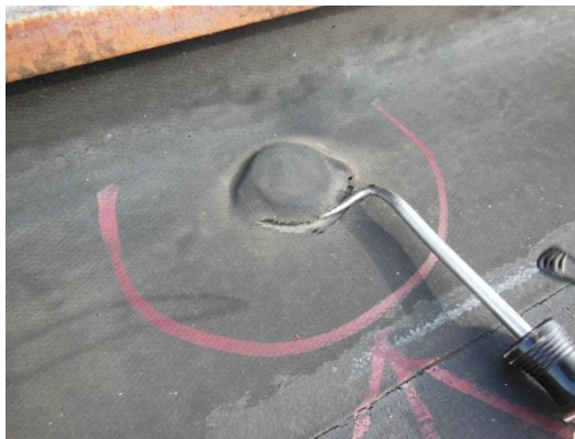
Self-adhering flashings are deteriorating over metal fastener plates; active water entry occurs.
