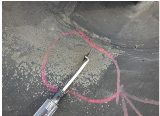
Small splits are observed at random locations in corner patches of skylight curb flashings.
