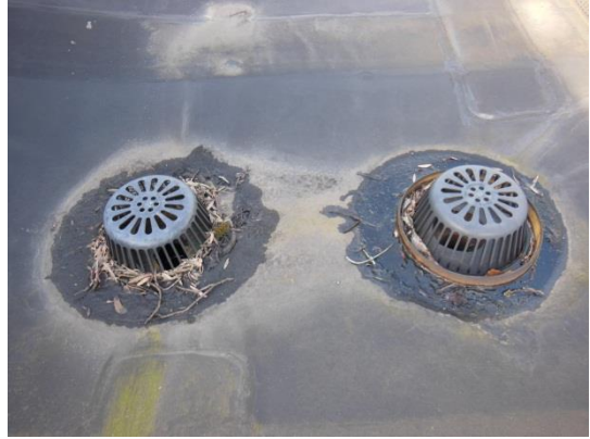
Drains are restricted by organic debris (typical condition).
