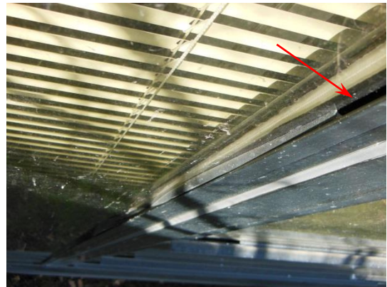
Weather stripping is missing from window frame.
