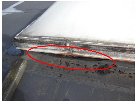
Curb flashing is open at top edge.
