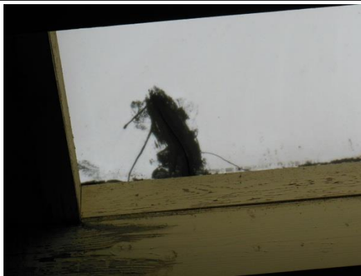
Interior view of skylight at active leak location.
