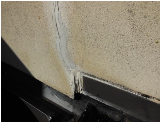
EIFS wall cladding has cracked.
