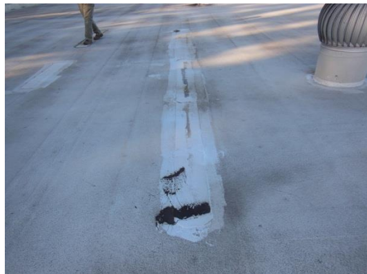
Previous membrane splits have been repaired with strips of modified bitumen material, and covered with aluminum coating.
