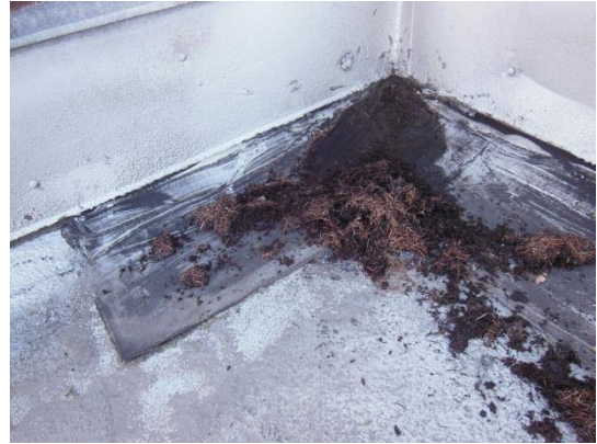
Repairs to perimeter base flashings and membrane in corners have delaminated.
