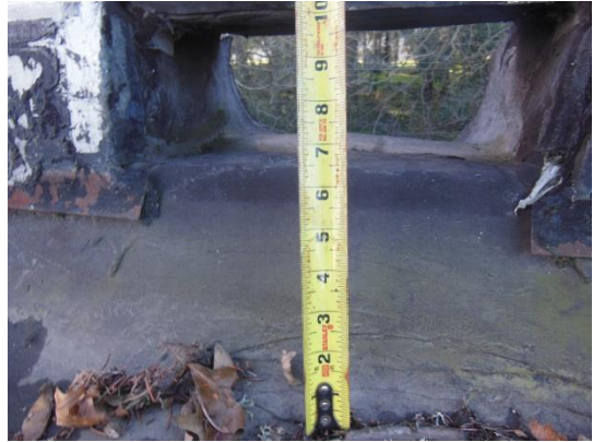
Overflow scuppers are set more than 6" above the finished roof surface allowing significant accumulation of water prior to activation.
