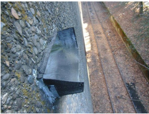
Scupper inserts have been fabricated out of modified bitumen material and may allow water to track back under the flashing.
