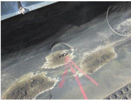
Flashing material has deteriorated over metal fastener plate at HVAC unit.
