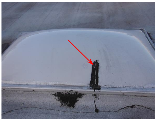
Skylights are failing. Several of the acrylic domes have large cracks.
