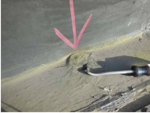
Flashing is deteriorated at fasteners plates around HVAC curb (active leak location).
