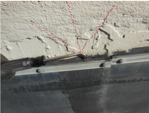
Termination bar is loose and sealant at top edge of flashing is deteriorated.
