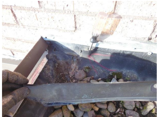
Perimeter flashings are open on Roof Area J.
