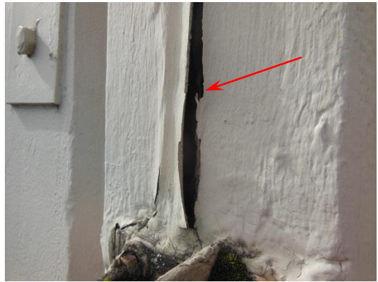
Sealant at vertical wall joint has failed.
