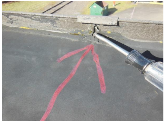
Membrane is disbonded from perimeter edge flashing.
