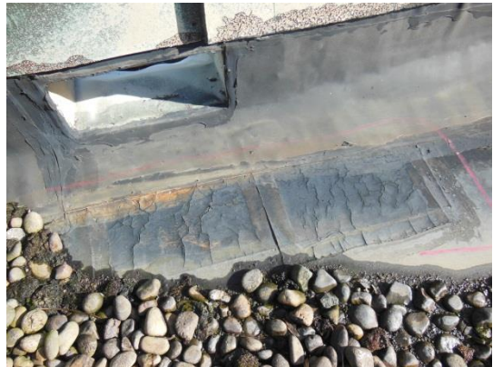
Perimeter flashing is deteriorating.
