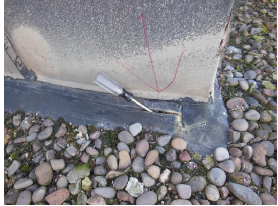
Curb flashing is open.
