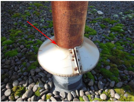
Top edge of storm collar is not watertight.
