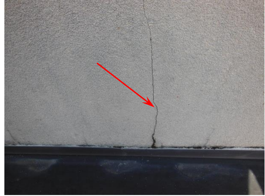
EIFS wall cladding is cracked in several locations on the interior of the wall.
