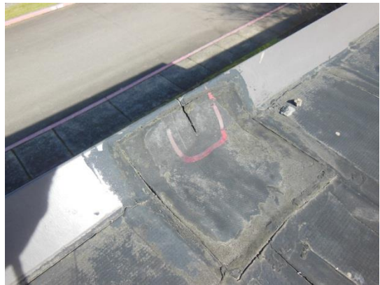
Flashing patches at joints in edge metal are splitting and may allow water entry.
