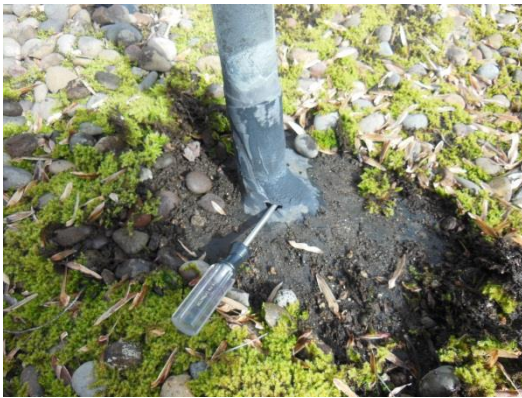
Field wrapped pipe flashings are deteriorated due to long term UV exposure.
