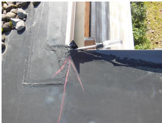
Corner of perimeter flashing has delaminated from edge metal.
