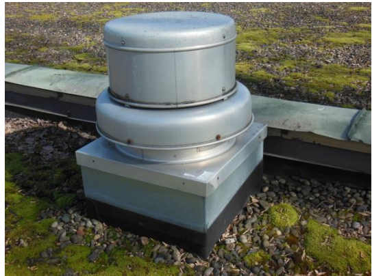
Curbed penetration flashing is not properly terminated.
