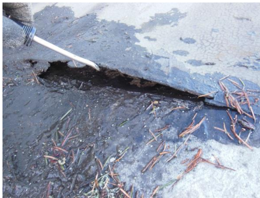
Repair membrane at drain locations is disbonded and can allow water beneath repair.
