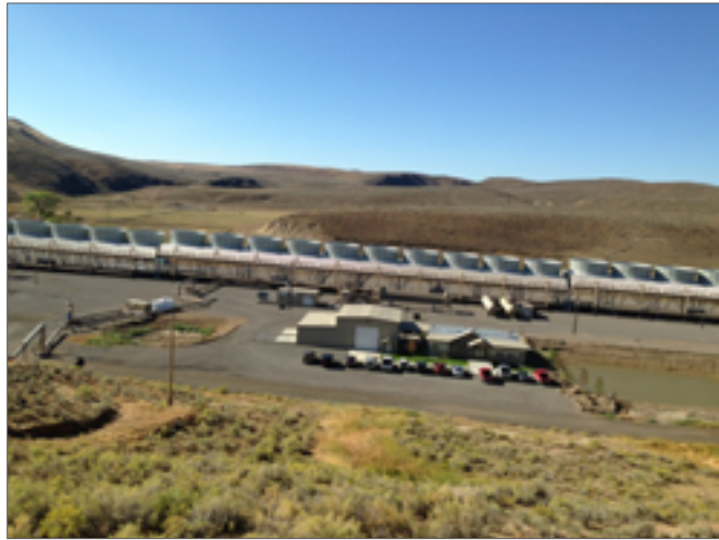
Neal Hot Springs, Malheur County, the first commercial geothermal plant in Oregon producing 21Megawatts.
