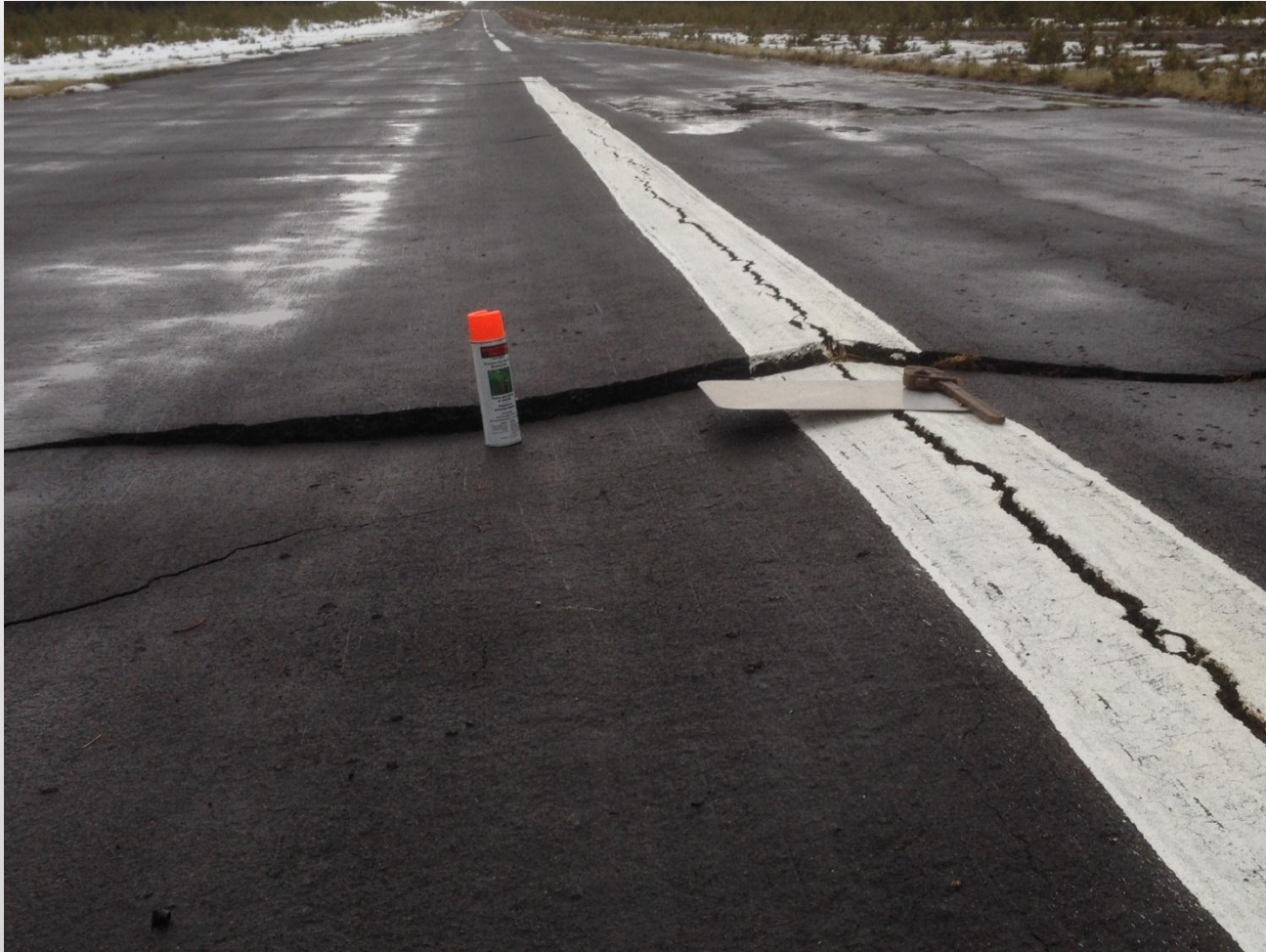
Crescent Lake - pavement damage
