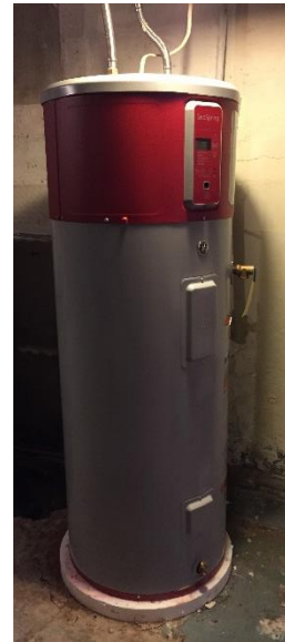
Electric Heat Pump Water Heater
