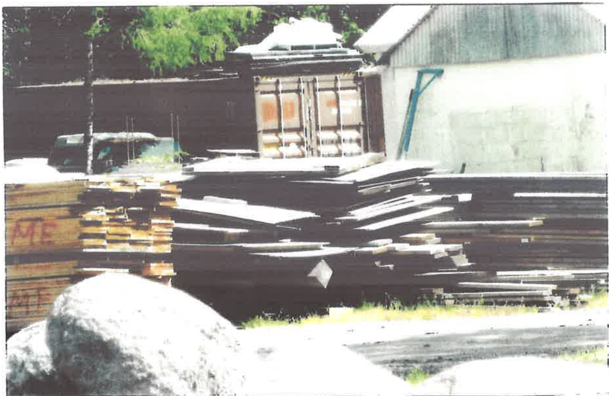
View of lumber and large metal storage containers (background) brought in and set up on site along E. Marmot Road.
