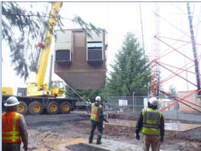
ODOT crew members guide the repurposed shelter into place on the new concrete foundation at McCully Mountain.
