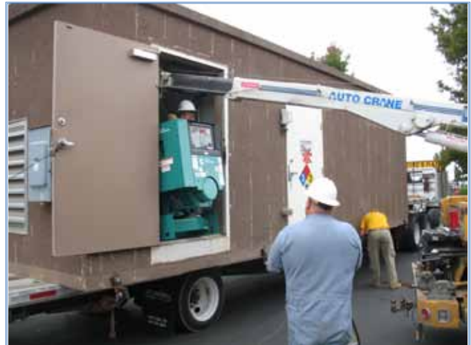
ODOT mechanic Jim Cooper maneuvers the crane lifting the generator into the shelter, while mechanic Jay Burkert helps guide it into place.
