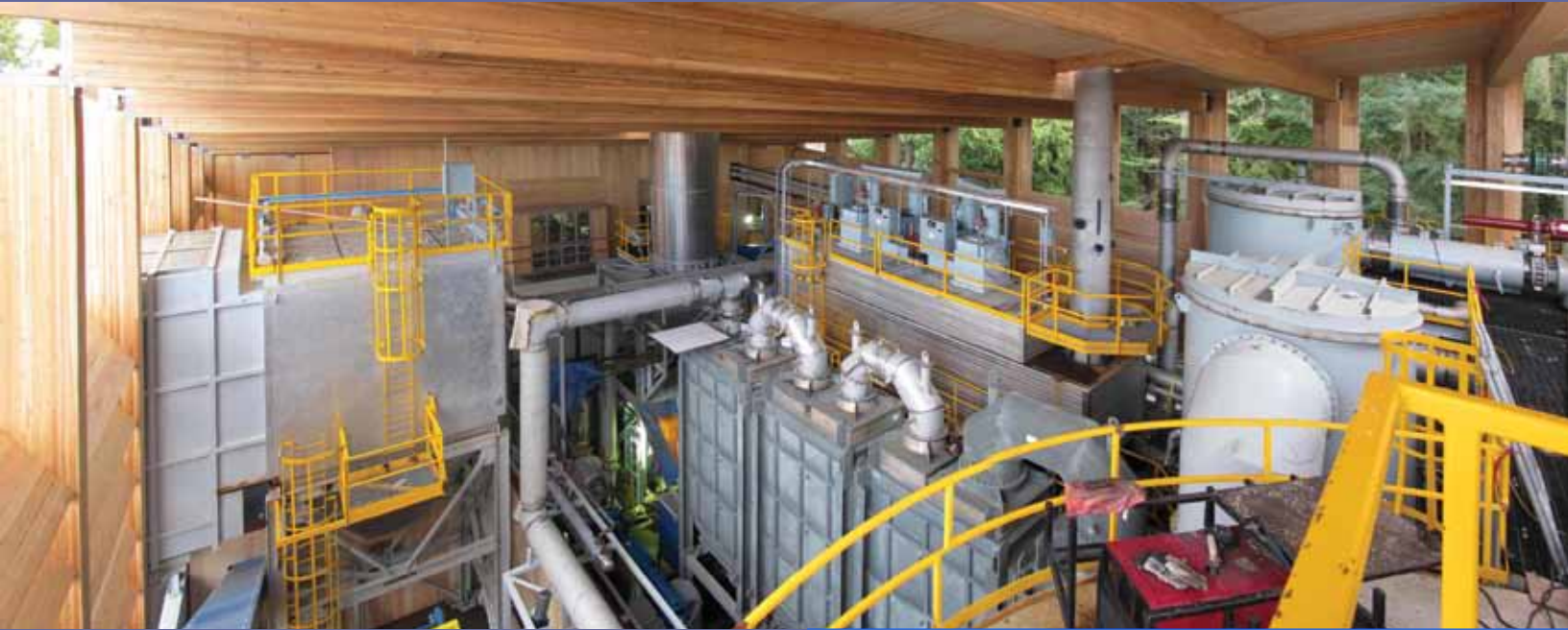
UBC Nexterra combined heat and power. Photo Credit: McFarland Marceau Architects Ltd.
