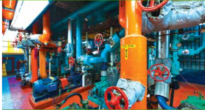
University of British Columbia district hot water system
