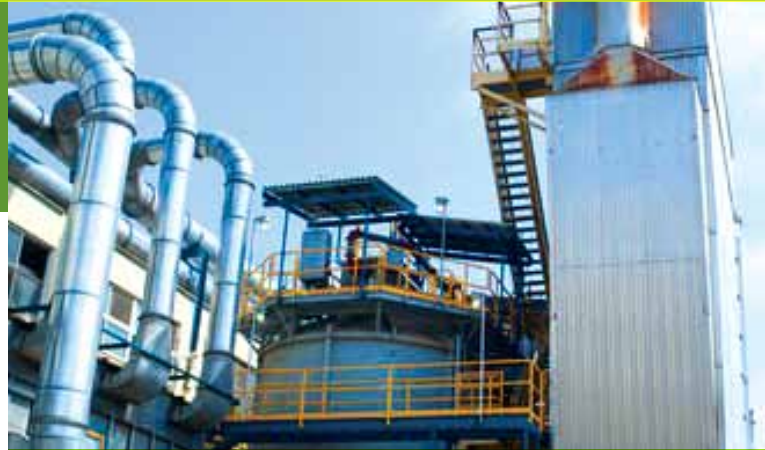
Kruger Biomass gasification. Photo credit: Nexterra Systems Corp.
