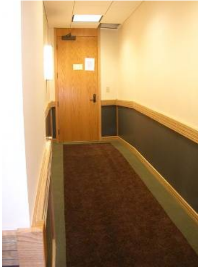
Figure: Common Error -This ramp provides access to the judge's bench from the rear; it lacks handrails. Additionally, the landing does not allow for someone to back up to get past the swing of the door or turn around if the door is locked or too difficult to operate.
