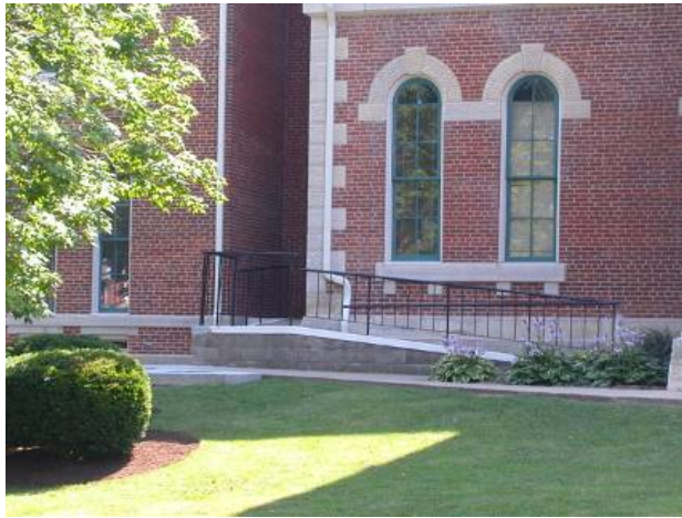
Figure: Common Error- This exterior ramp is located so that it provides access to a back door that is not visible from the outside.
