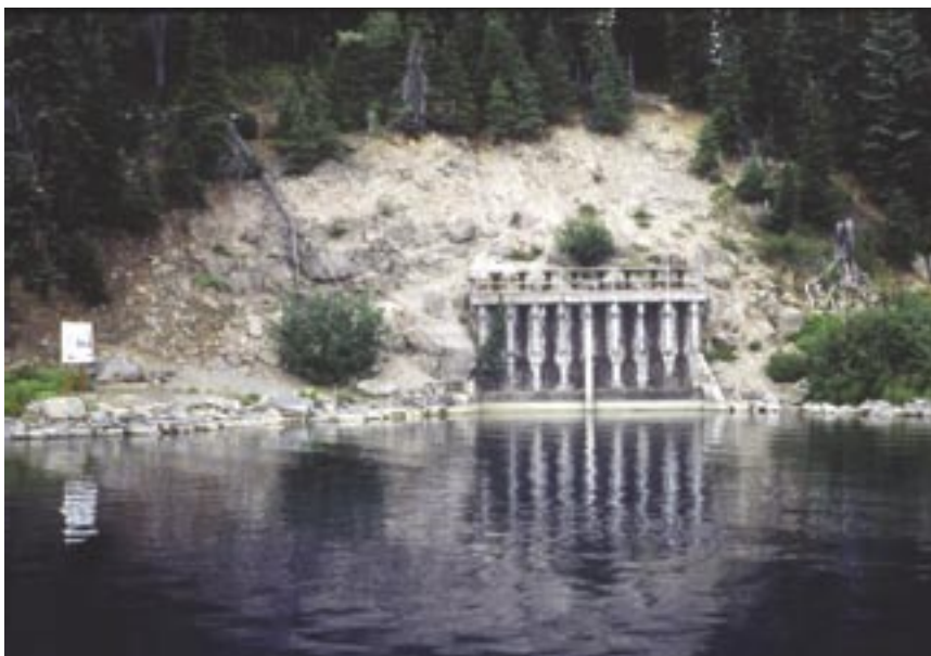
Figure 4. Klov Dahl tunnel entrance and head-gate at Waldo Lake, August 1990. Photo by author.
