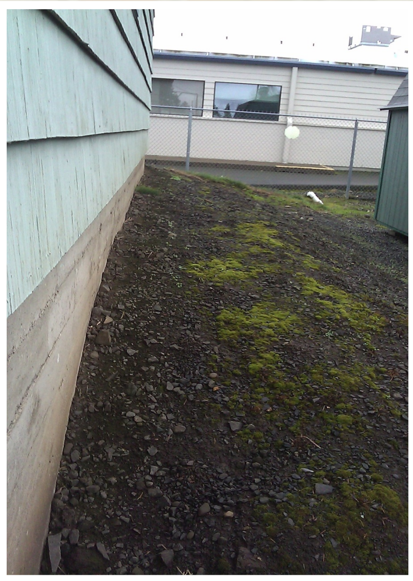
Dirt fill being used to prevent foundation wall from tipping out further.
