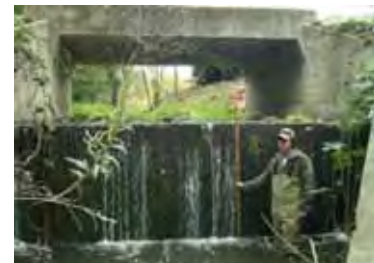
Fish Passage Barrier on Lazy Ck.
