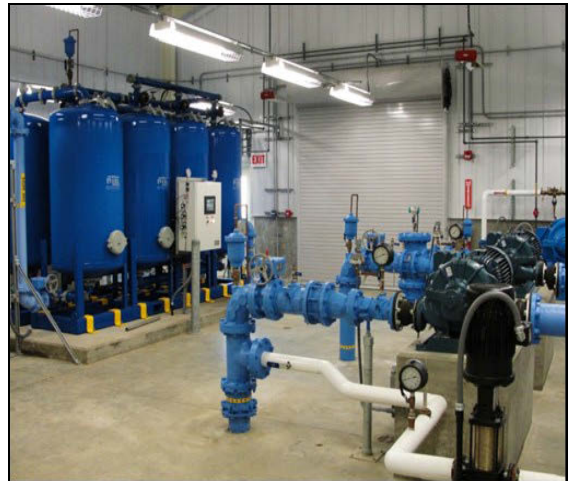
Photo (Right): Water supply system, water treatment plant.
