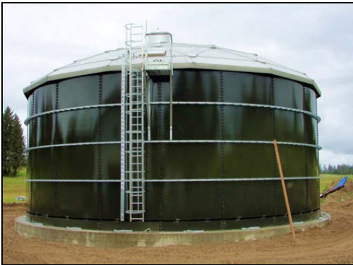
Photo (Above): 426,000 gallon storage reservoir for Water Supply System.
