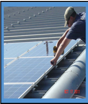
Photo (Above) Hire Electric employee installing 235 watt panels. This fastening system is specifically designed for Butler roofs.
