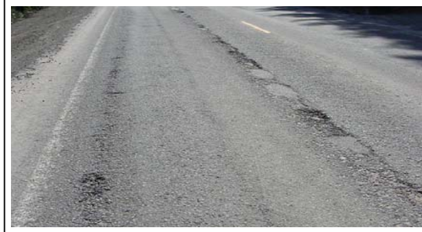
Pavement Condition: Poor
