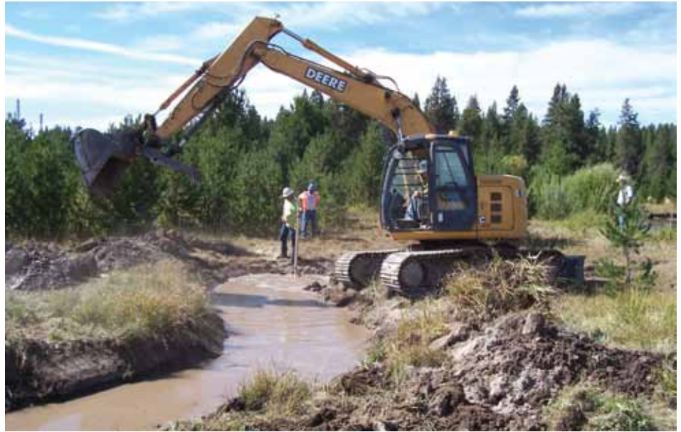
Rebuilding a stream channel to restore connectivity for bull trout, made possible by CFLR. © Craig Bienz
